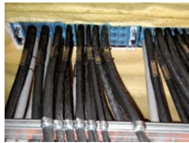
Fig. 7 Correct cable sealing with Roxtec
