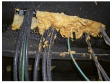
Fig. 6 Incorrect cable sealing
